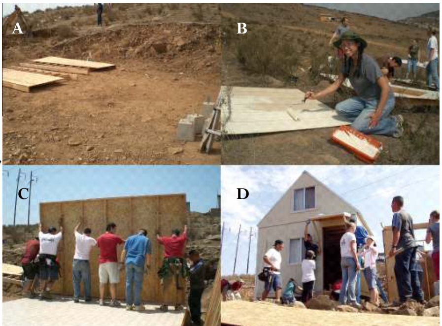
A new home is built. A: The empty plot of land before construction began. B: Jennifer Jung paints with a smile. C: The first wall is raised. D: Putting on the finishing touches to the house.
